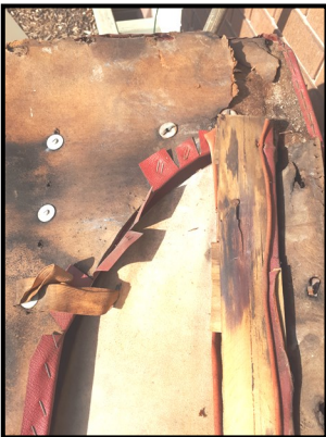
Rotted Door Cards
